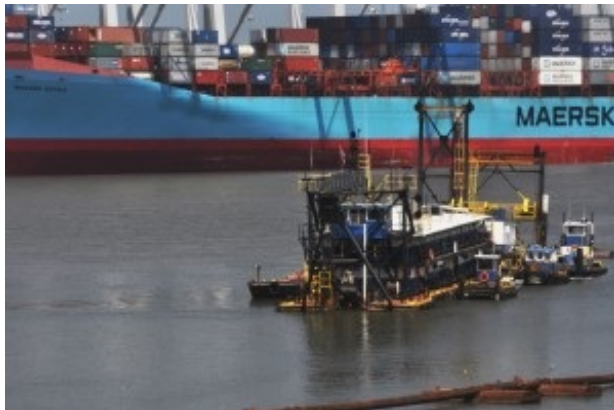
The Dredge Brunswick performs maintenance dredging in the Savannah Harbor, Savannah, Ga. The U.S. Army Corps of Engineers Savannah District oversees maintenance of the harbor. U.S. Army Corps of Engineers photo by Billy Birdwell
