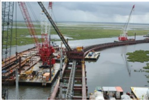
Construction continues on the Inner Harbor Navigation Canal Surge Barrier, dubbed the "Great Wall of Louisiana," is one of the main perimeter structures of the Hurricane and Storm Damage Risk Reduction System. Photo courtesy of the U.S. Army Corps of Engineers
